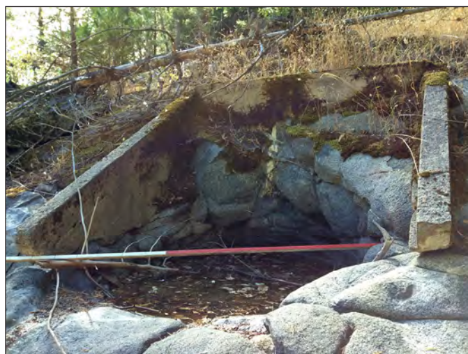
Figure 3. Large basin at White Hall springs on south side of South Fork American River (see fig. 1 for location), showing mortar walls built to increase capacity. Basin is about 1.5 m wide (red half of rod is 1 m long).
